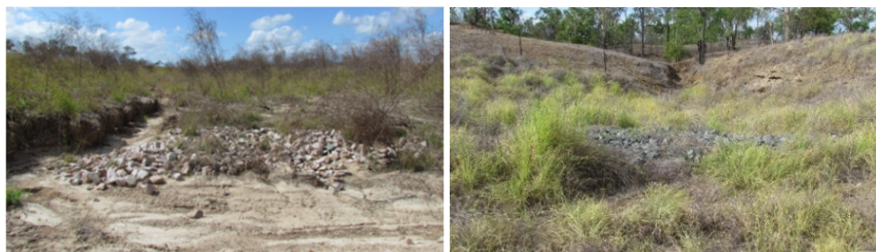
Figure 5. Poor and good porous rock check dam implementation. Image left; outflanking of PCD abutments. Image right; constructed as per design with no outflanking.
